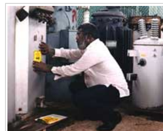
Labelling transformers containing PCBs Source: US federal Government
