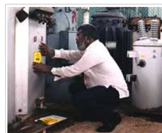
Labelling transformers containing PCBs
