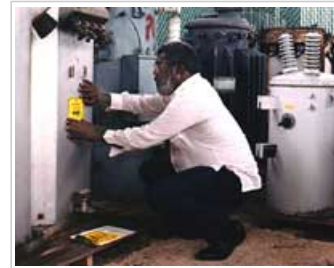
Labelling transformers containing PCBs
